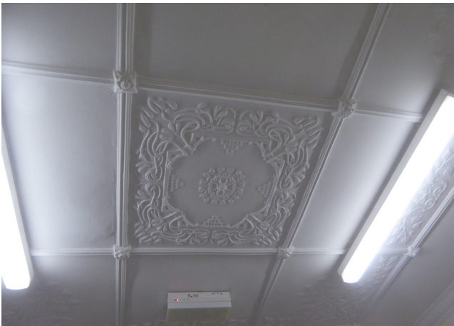
Figure 3.12 Existing decorative plaster ceiling within the lounge space, note the fluorescent lighting and fixed services (Item 6C).
